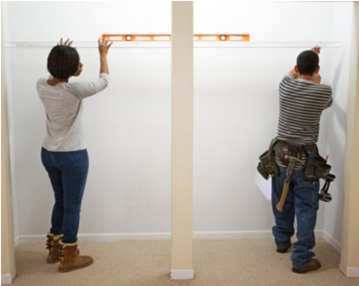
Takeisha Washington and Jose Vargas building shelves for a family of three excited about moving in.
