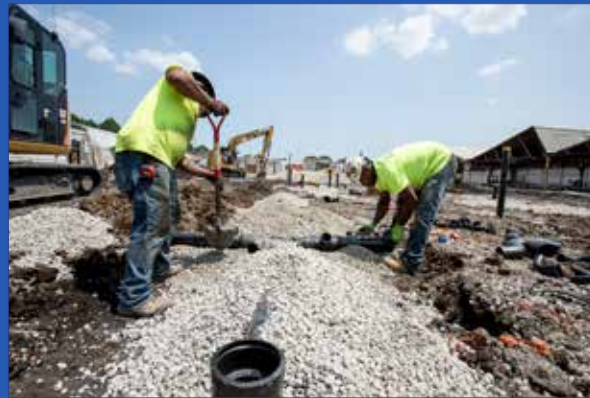
CED Food LLC took the next step in bringing Amped Kitchens to Chicago's Belmont-Cragin neighborhood by breaking ground on the Northwest Side project in July 2019.
