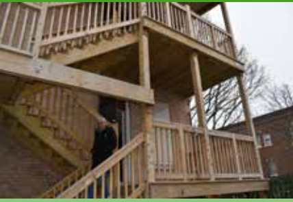
One of the major accomplishments of RPT Development's rehab is completely rebuilding the outside balcony and stairs.
